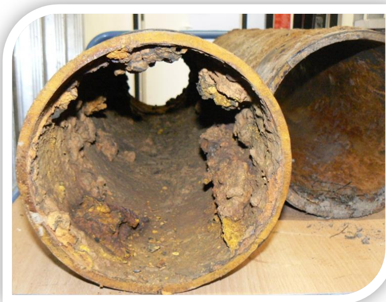
Figure 11: Development of rust and microbial growth in a cast iron pipe. Here, example on a public main pipe. (Source: KWR)
